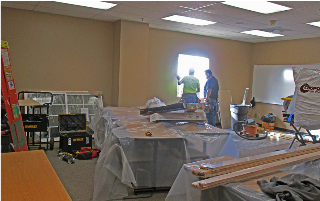
Contractors installing a window in the Archival Seminar Room, newly outfitted with updated digital equipment and soundproofed, where archivists provide instruction to faculty and classes in using primary sources using Archives' collections.
